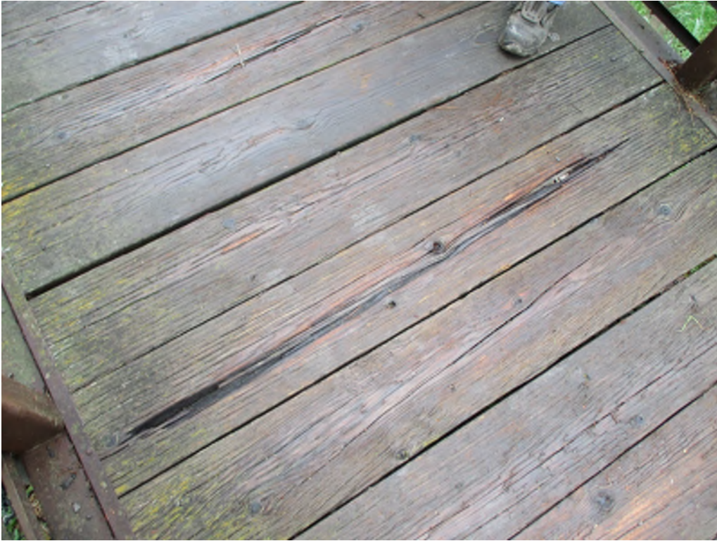
Image 9: Cracked and Rotted Floorboard
