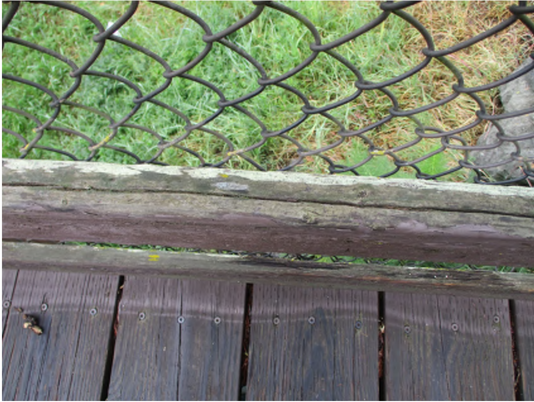
Image 7: Handrail Member Condition
