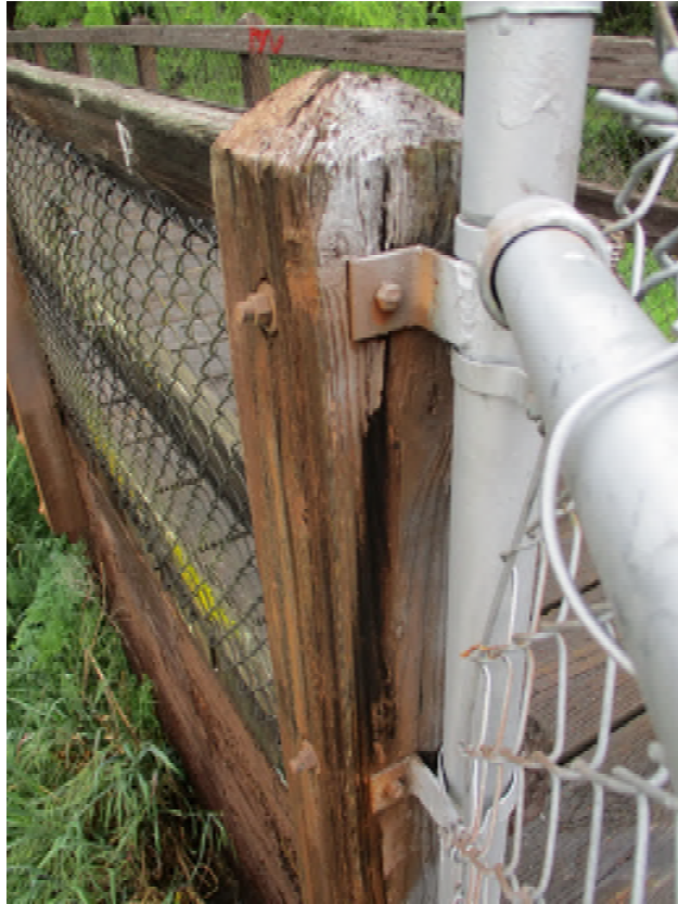
Image 11: Handrail Post Condition
