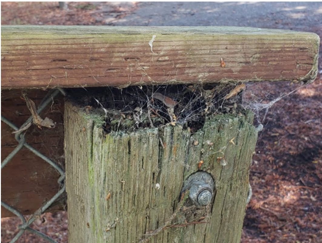
Image 10: Handrail Post Condition
