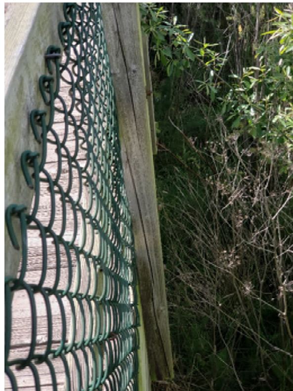
Image 12: Handrail Post Condition
