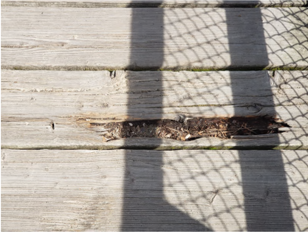
Image 9: Cracked and Rotted Deck Board
