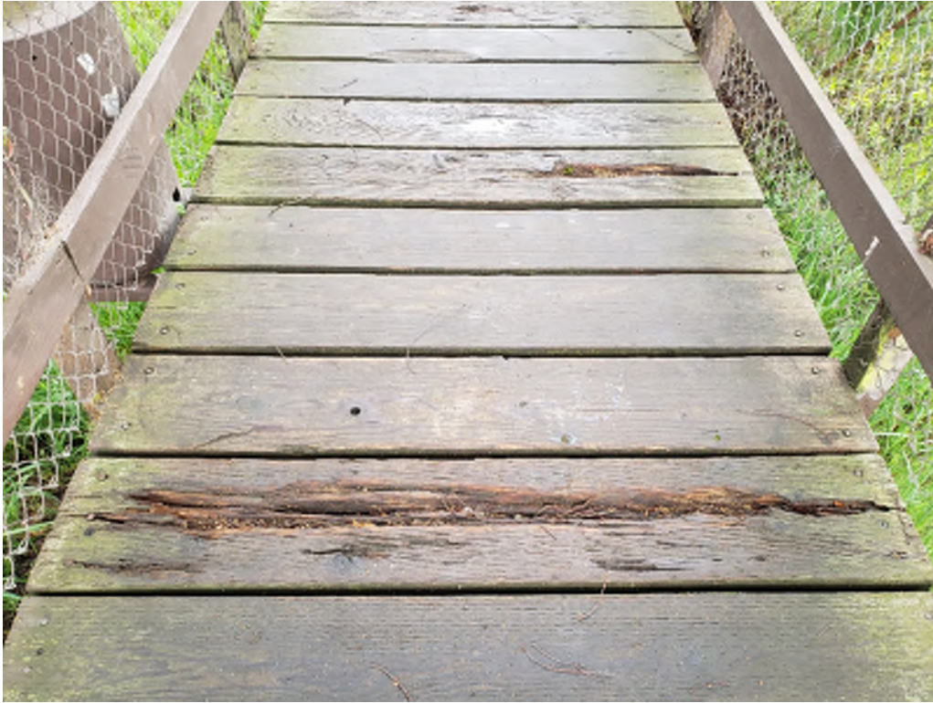
Image 9: Cracked and Rotted Deck Board
