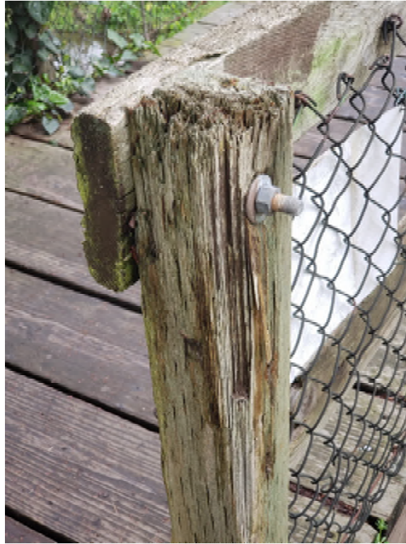
Image 9: Deteriorating Handrail Post
