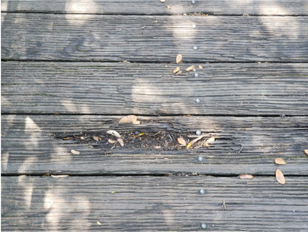
Image 9: Cracked and Rotted Floorboard
