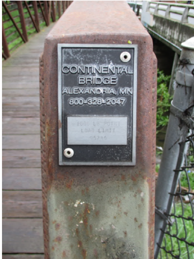
Image 17: Bridge Capacity Plaque
