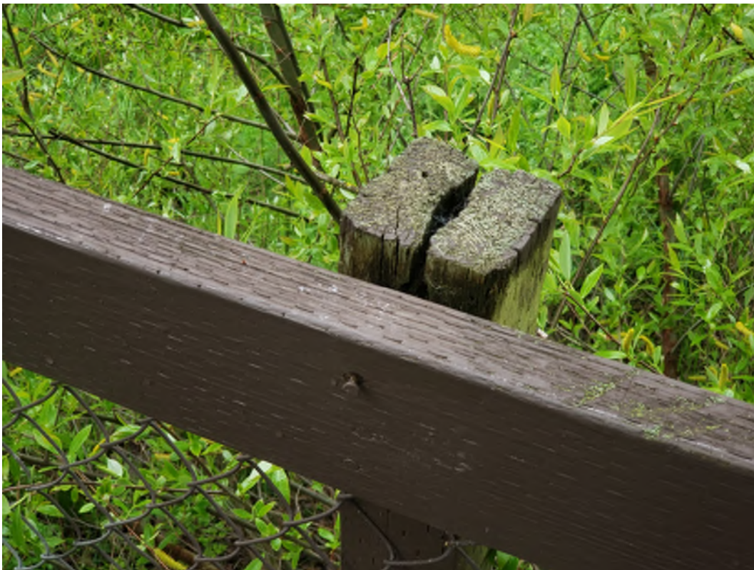
Image 12: Handrail Post Condition
