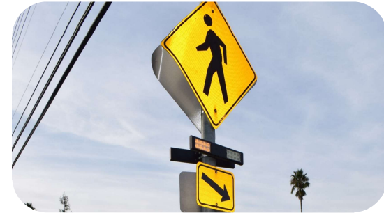
Rectangular Rapid Flashing Beacon
